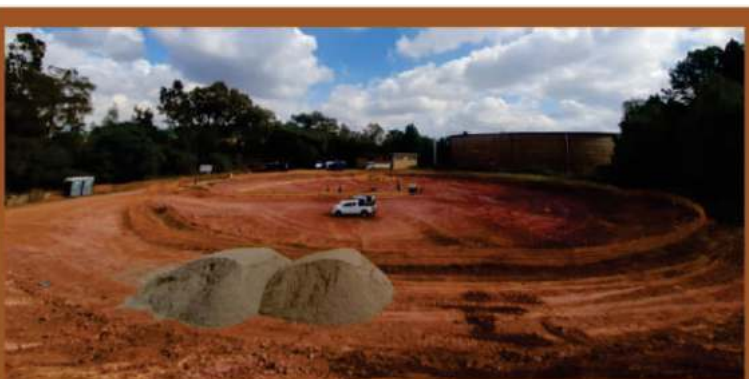
The National Department of Public Works and Infrastructure is currently undertaking the installation of bulk and internal infrastructure at the Salvokop mixed-use precinct project within the ambit of the Tshwane Inner City Regeneration Programme.
