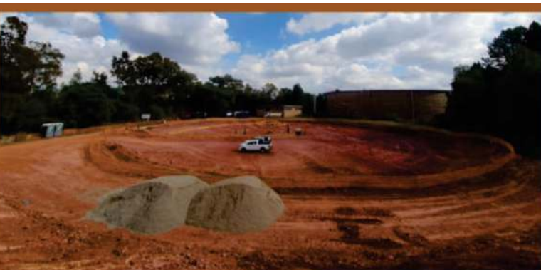
The National Department of Public Works and Infrastructure is currently undertaking the installation of bulk and internal infrastructure at the Salvokop mixed-use precinct project within the ambit of the Tshwane Inner City Regeneration Programme.
