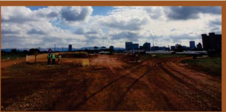
The construction of Phase 1A: Bulk Civil and Internal Engineering works is currently in progress with a number of local residents and SMMEs from the nearby community already employed on the project.
