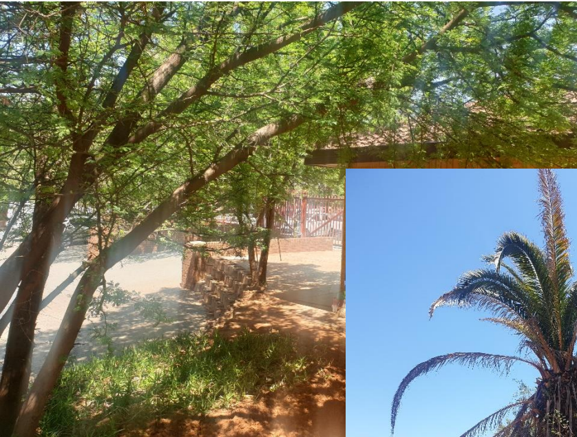
Prune branches of tree hanging over roof. (Tree 5 of 5)
