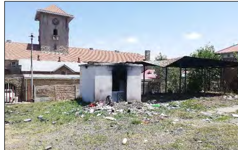
Picture 4: Looking north west towards the existing carport and outbuilding which are present.
