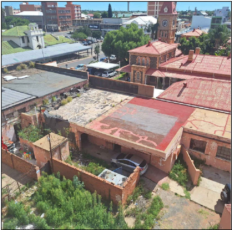
ROOF PHOTOGRAPH - HIGHLIGHTING DEFECTS NOT TO SCALE
