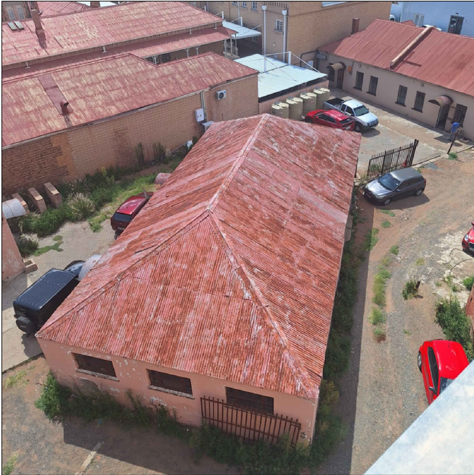
ROOF PHOTOGRAPH - HIGHLIGHTING DEFECTS NOT TO SCALE
