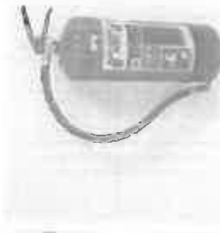
FIRE EXTINGUISHERS: Fully maintained F/E located to OHS standards
