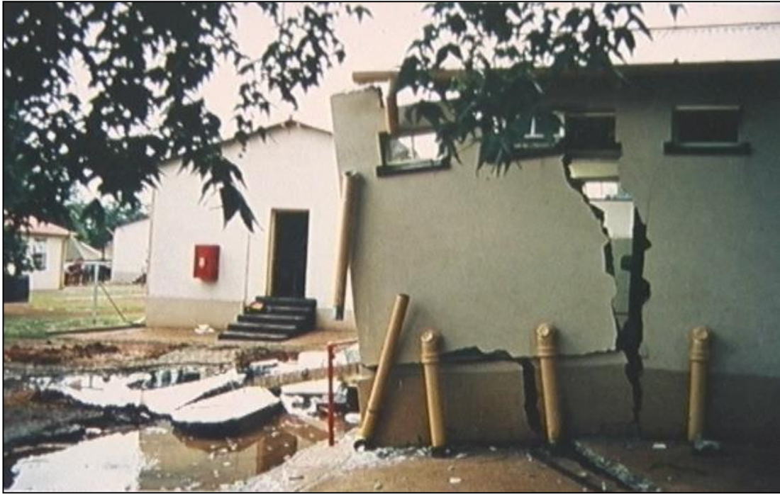
PLATE 9: Building movement as result of subsidence formation
