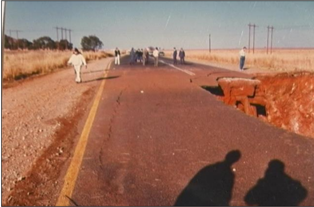
PLATE 3: Sinkhole on highway as result of leaking water pipe
