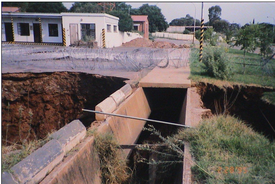
PLATE 2: Sinkhole as result of leaking stormwater canal
