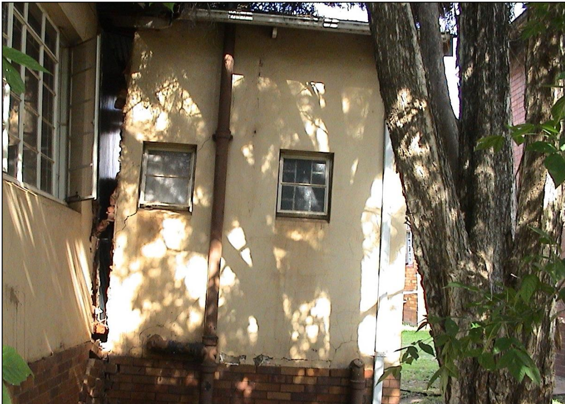
PLATE 8: Building movement as result of subsidence
