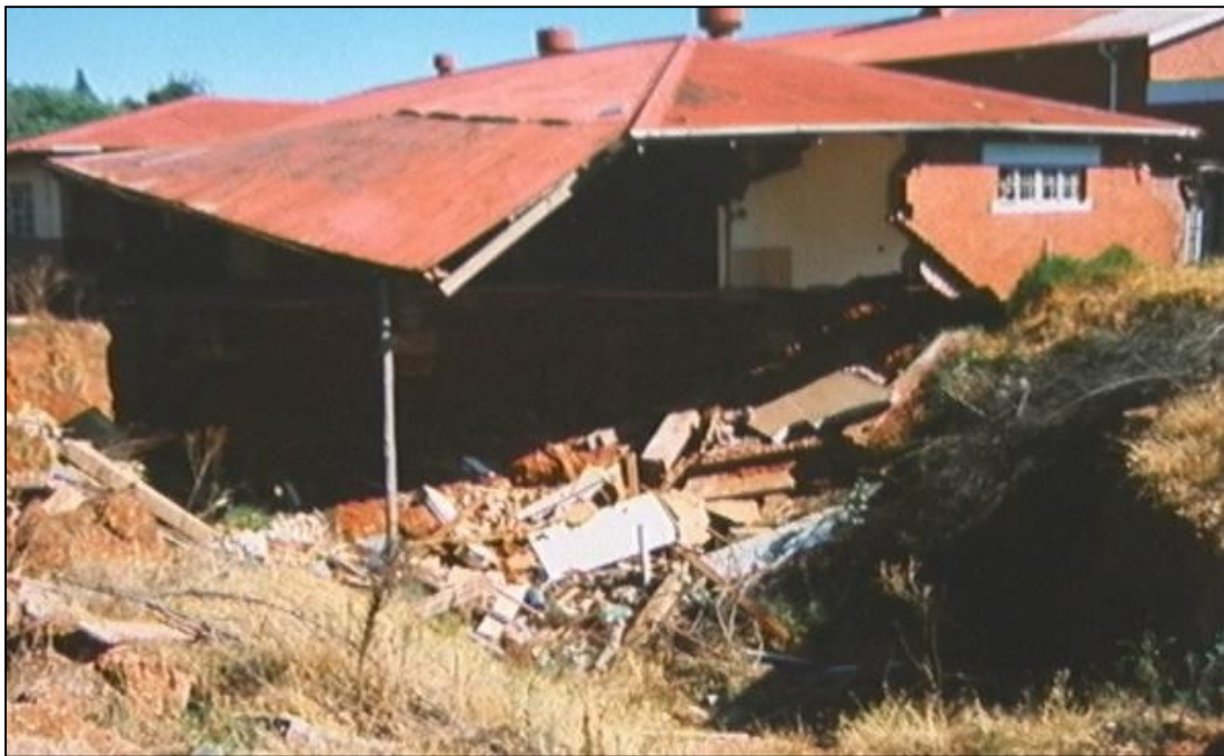
PLATE 6: Sinkhole as result of leaking wet service
