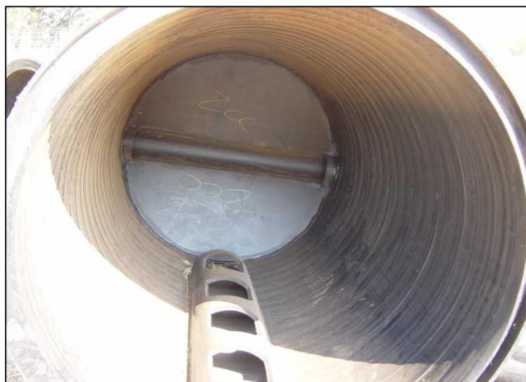
HDPE SEWER MANHOLE OF STRUCTURED WALL HDPE PIPE (INSIDE)
