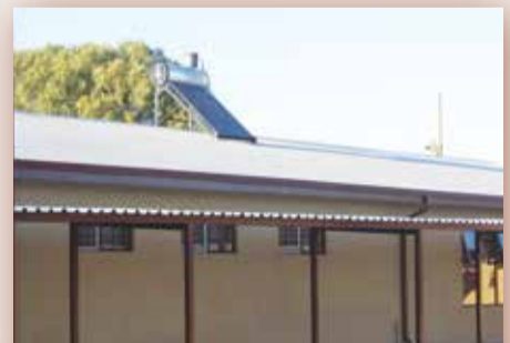
Solar panel installed to the building
