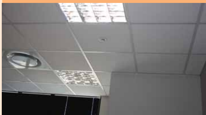
Sensors that automatically switch lights on when one enters the room
