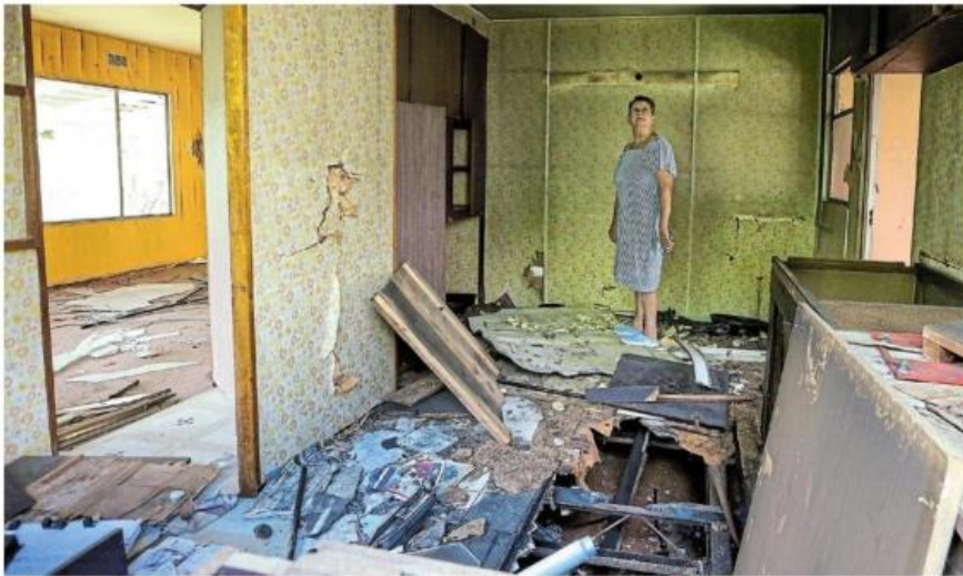
IN RUINS: The defunct Rocklands satellite police station, which once housed a fully operational client services centre, was declared uninhabitable in 2021 by the national government. Resident Marie Swanepoel surveys the damage inside the derelict structure. Pictures: WERNER HILLS
