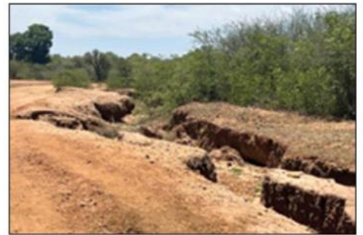
Erosion along the shoulder of the D3668 makes the road very dangerous to drive on. Photo: Roads Agency Limpopo.
