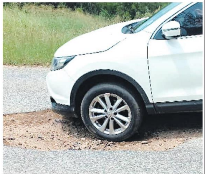
A car shows how deep the potholes are.
