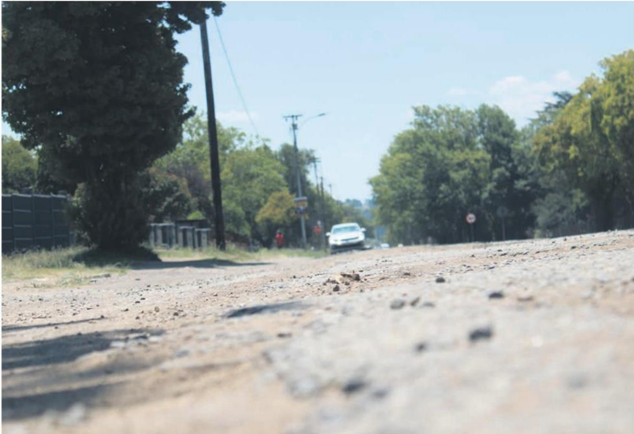
Motorists have to veer into opposite lanes in Clerq Street, Bethal, to prevent hitting potholes.
