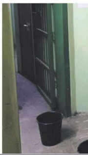
Buckets have been placed to collect water dripping outside the holding cells at the Pietermaritzburg Magistrate's Court.
