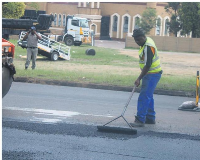
A workers is repairing the holes on Beyers Naude Drive and Handel Street in Standerton.
