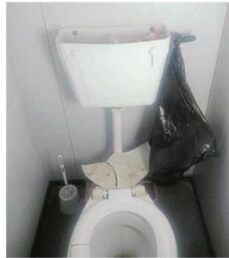
UNHYGIENIC CONDITIONS: A female bathroom in the Ngqamakhwe temporary police station has a broken toilet and uses black plastic bag as a sanitary bin. Picture: SUPPLIED
