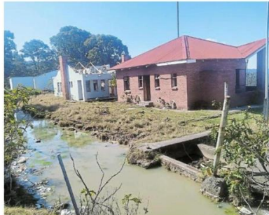
FINDING REFUGE: Homeless people have occupied one of the vandalised Ngqamakhwe police station buildings. Picture: MKHUSELI SIZANI
