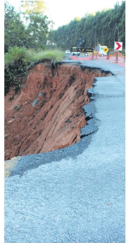
Part of the damaged road on the R40 next to Klipkopjes Dam.
