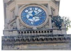
A FIG tree stands sentinel next to the clock tower of the Durban post office, one of the oldest buildings in the CBD. However, experts say the tree could cause considerable damage to the building, which has been observing the hustle and bustle of life in the city centre for more than a century. | DOCTOR NGCOBO African News Agency (ANA)
