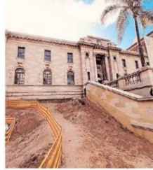
THE DURBAN High Court redevelopment and renovation project by the Department of Public Works and Infrastructure is 55% complete. | SUPPLIED
