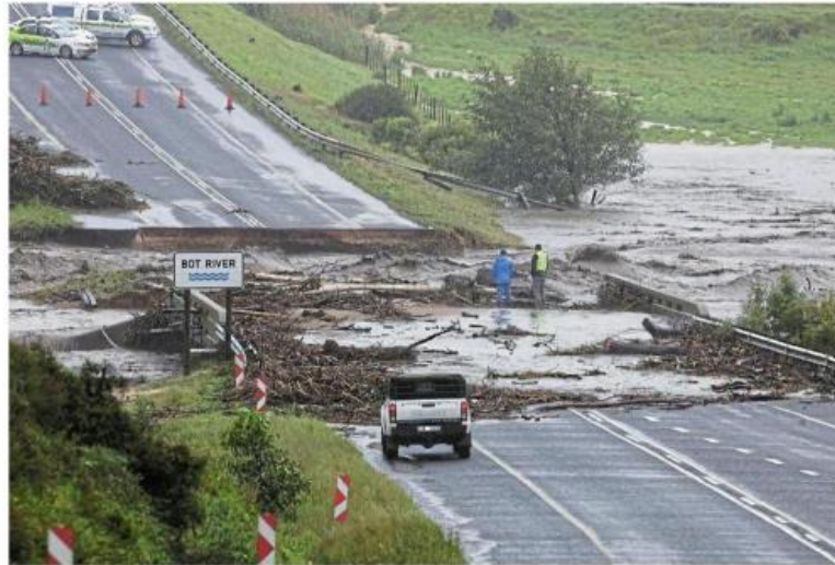
Swept away: A view of a damaged road between Botriver and Caledon on Monday after heavy rains in the Western Cape. Several rivers broke their banks, destroying infrastructure, causing electricity outages and flooding homes and farmland in Cape Town, the Overberg, Overstrand and the Winelands. /Reuters
