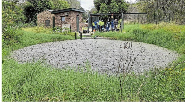
An overflowing sewage dam at the Drakensig wastewater treatment works in Hoedspruit. /SUPPLIED
