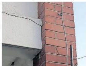
THE crumbling walls of Ferndale Primary School are a cause for concern. | SUPPLIED.
