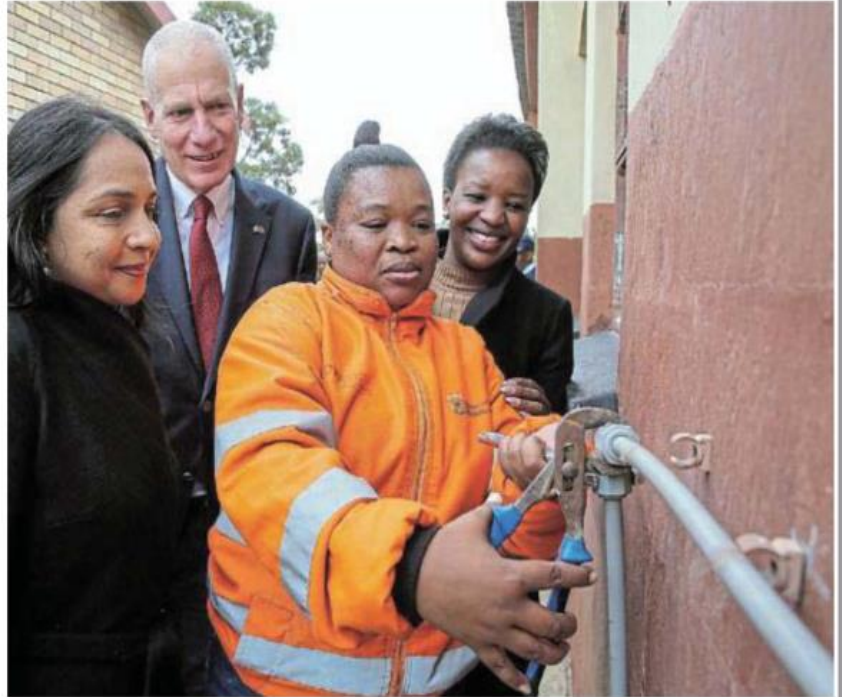
ALL SORTED: Pendla Primary School in New Brighton is part of a pilot programme, where along with the fixing of toilets, community members were trained as plumbers to maintain them. Back, from left, National Business Initiative CEO Shameela Soobramoney, US consul-general in Cape Town Todd Haskell and Business Leadership SA CEO Busi Mavuso look on while Amanda Dyasi, front, shows the skills she has learnt
