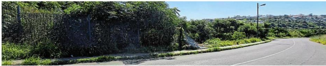
RESOURCE RAMMED: Newly constructed fence in Buffalo Flats, paid for from the ward 19 budget last year, was damaged last week because of vandalism. Picture: TAMMY FRAY
