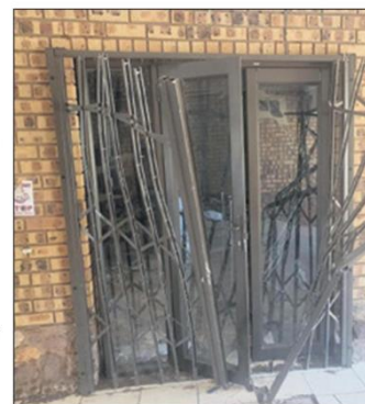
One of the vandalised buildings at the Mphephu Resort. Photo: Lutendo Bobodi.
