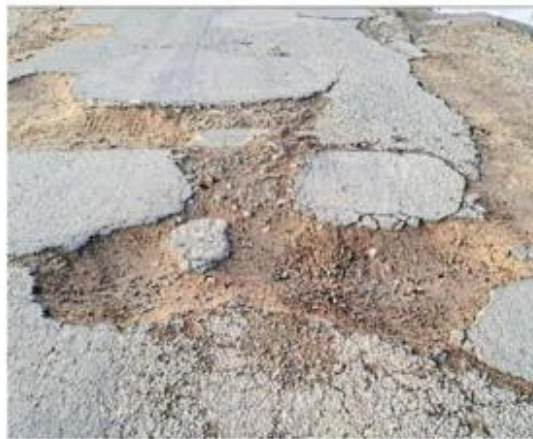
Pay up: A former North West public works MEC must pay the costs of a motorcyclist injured on a road in need of repair. /Supplied
