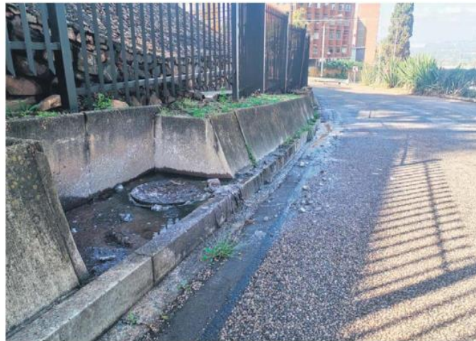
FOUL SMELL. Sewage overflows from a burst sewage pipe outside Hoërskool Wonderboom in Pretoria. Picture: Marizka Coetzer
