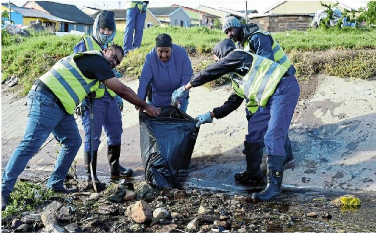
WET WORK: Getting their hands dirty in the stormwater infrastructure cleaning project in Bethelsdorp yesterday are, from left, roads and transport political head Bradley Murray, councillor Noline Moodley, Keithon Goliath, Alberto Damons and Rowan Schutte Picture: EUGENE COETZEE
