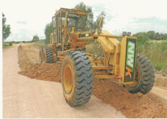
Agribusiness NWK recently embarked on the second phase of road rehabilitation in North West to provide passable roads to grain producers in the 2022/23 harvesting season. Most of the gravel roads leading to its silos in the province had become virtually impassable due to bad weather and poor maintenance. NWK
