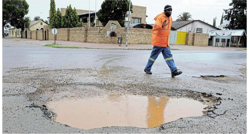
A pedestrian walks past a pothole in front of the ANC's North West head office along a busy main street in Mahikeng. /TIRO RAMATLHATSE
