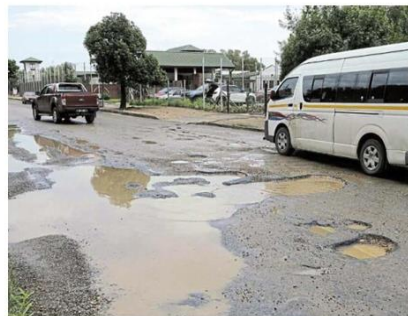
Motorists navigate a pothole on Carrington Street in Mahikeng. /TIRO RAMATLHATSE
