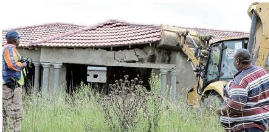
DOWN IT GOES: This house near one of Mthatha's affluent suburbs was illegally built on prime land.
