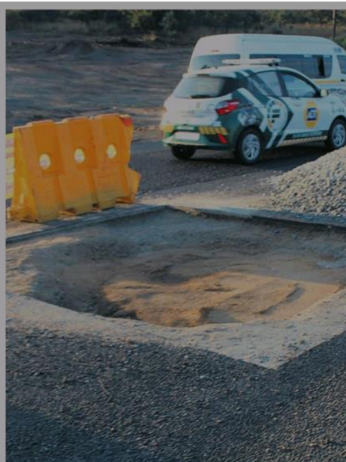
Laboratory results from soil density tests at the sinkhole have been received, and the repairwork appears to have commenced. > Photo: Tumelo Waga Dibakwane
