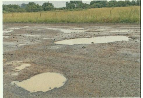
Dilapidated infrastructure costs South African farmers millions of rands as they struggle to transport their produce on potholed rural roads. ANNELIE COLEMAN
