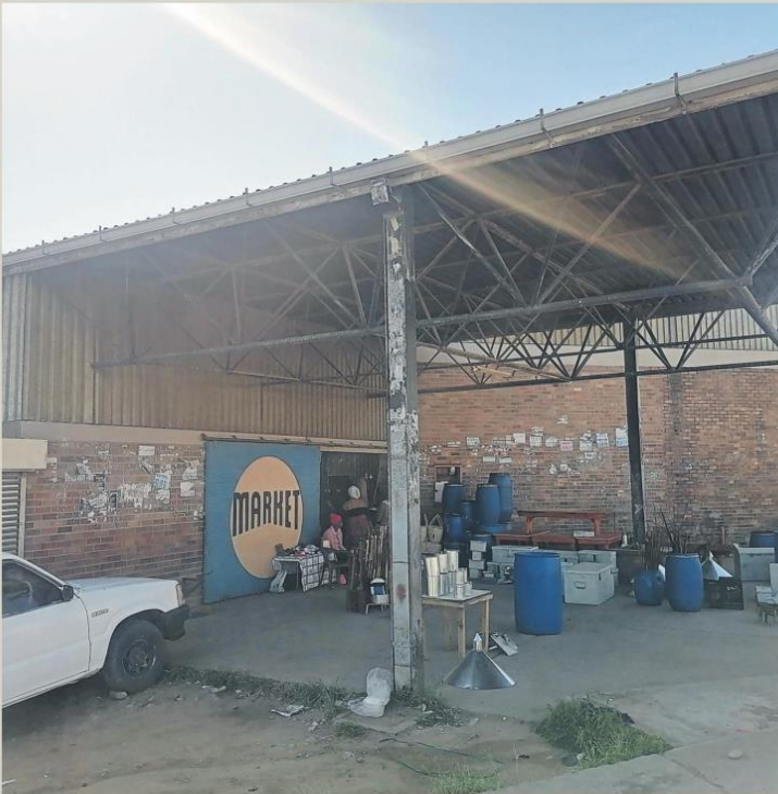
The Kwantozonke Market that is currently being renovated by the King Sabata Dalindyebo Local Municipality. PHOTO: LUVU CAKATA
