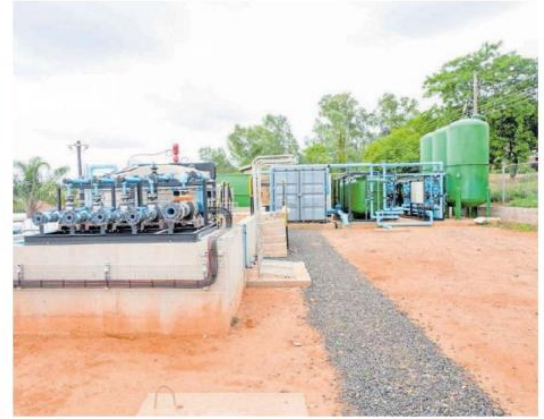
The newly-launched Bronkhorstbaai water treatment plant.
