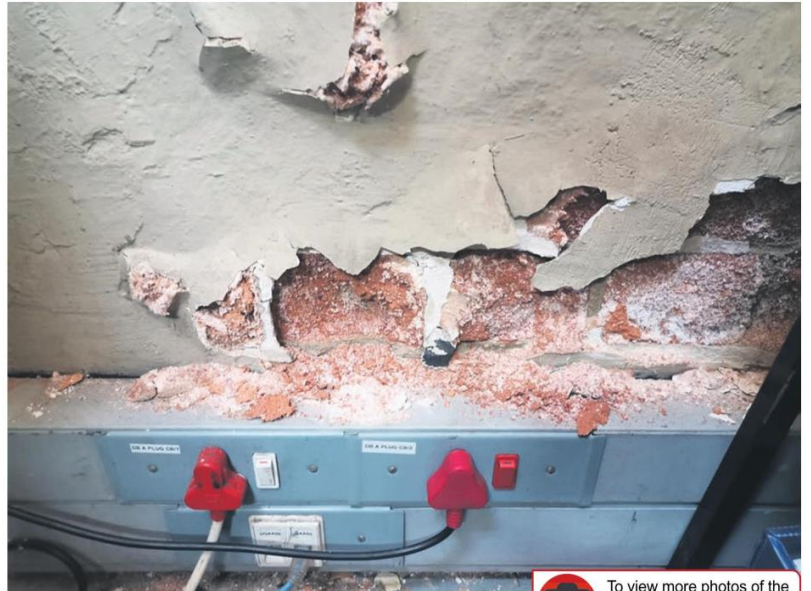
Cleaners are reportedly struggling to keep up with the amount of plaster and paint flaking off the walls of the police station.
