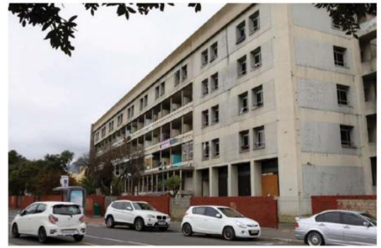
THE Helen Bowden Nursing Home building houses more than 800 illegal occupants. | BRENDAN MAGAAR African News Agency (ANA)
