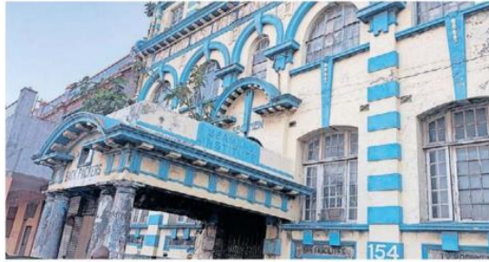
THE SEAMEN'S building, one of the old, dilapidated government buildings that was used by seamen until the end of the century, is one of the city's eyesores. | Supplied
