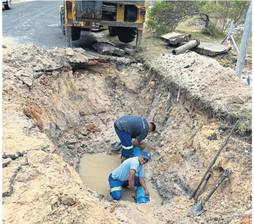
A pipe burst caused a water outage of up to seven days in Da Gama Park. PHOTO: SUPPLIED
