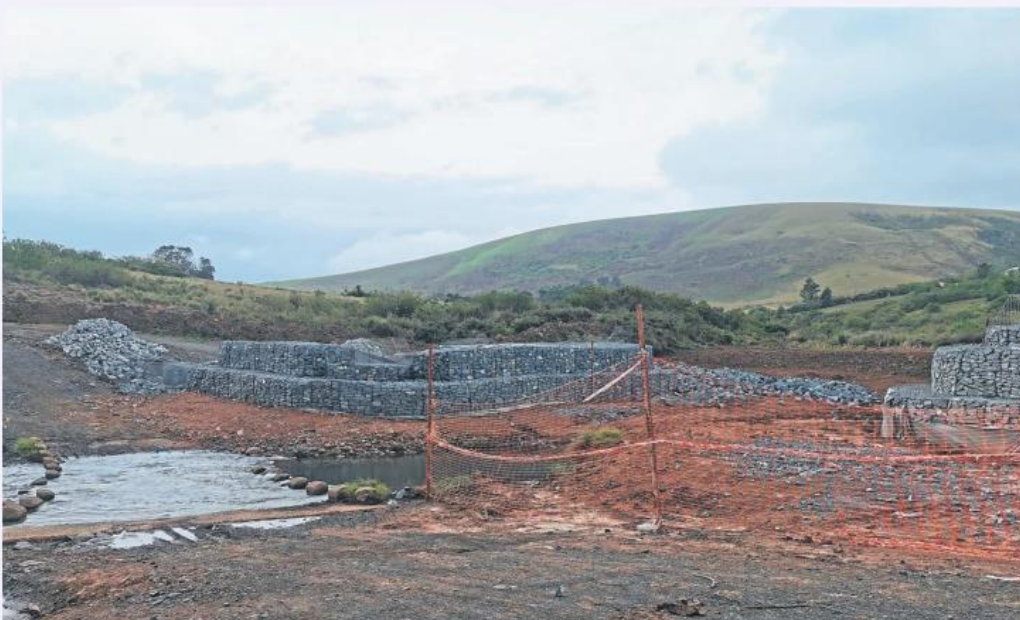
One of the bridge construction sites that Public Works and Infrastructure minister Sihle Zikalala visited in Port St Johns.
