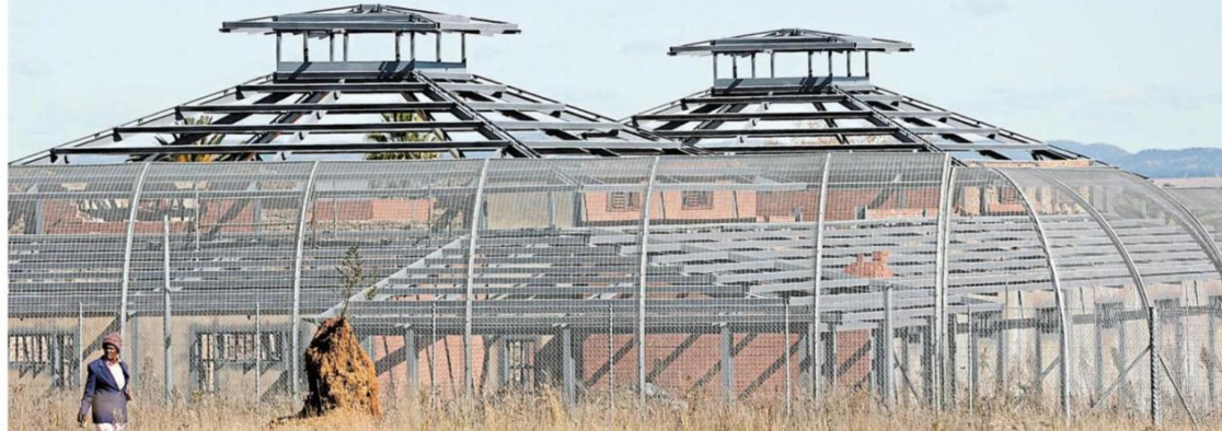
Edwin Sodi's company was supposed to upgrade this 65-bed correctional services facility to a 240-bed prison. /PHOTOS/ THULANI MBELE
