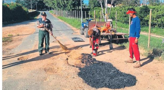
CWDM and DFW is seen jointly fixing potholes in the Paarl rural area.
