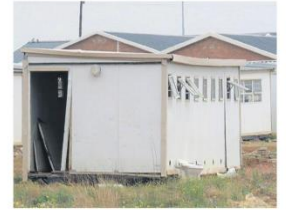
The ablution facility at which the incident happened.
