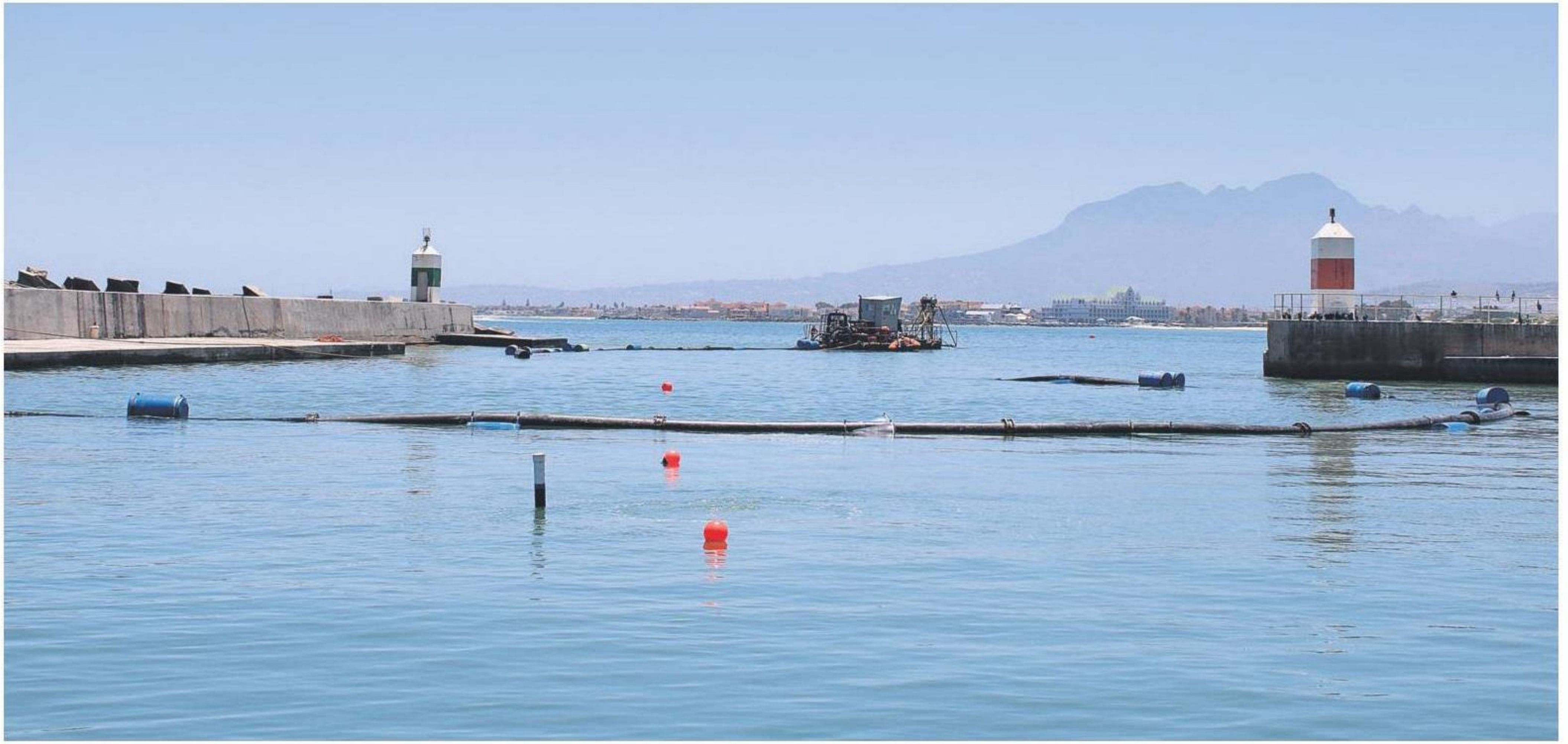
Dredging activity to deepen the seabed at the Gordon's Bay Harbour is nearing completion ahead of the holiday season. Photo: Yaseen Gaffar
