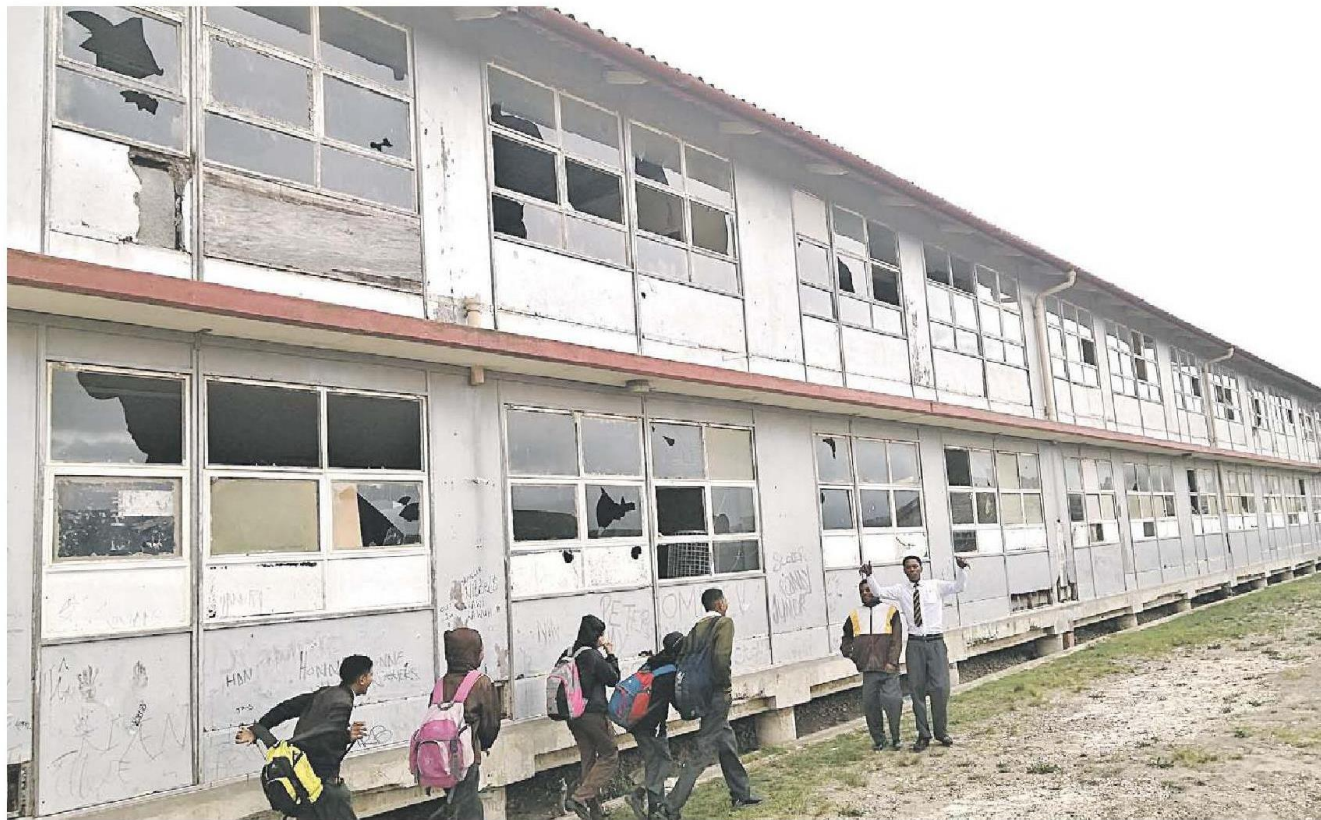
UNDER SIEGE. Arcadia Secondary School in Port Elizabeth is crumbling. Picture: Mkhuseli Sizani
