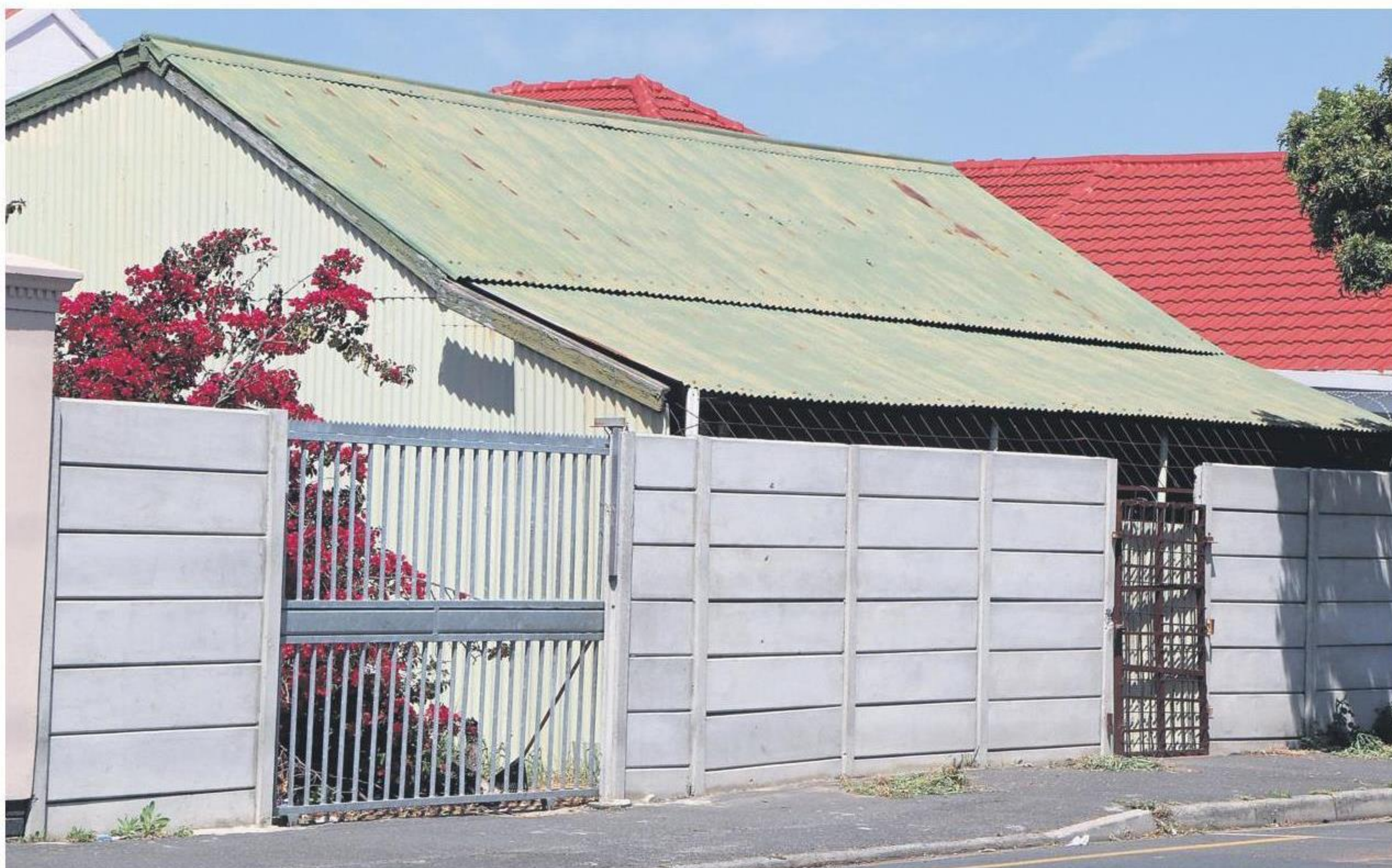
The house located at 24 Beaufort Street is a concern for residents. PHOTO: TARRYN-LEIGH SOLOMONS
