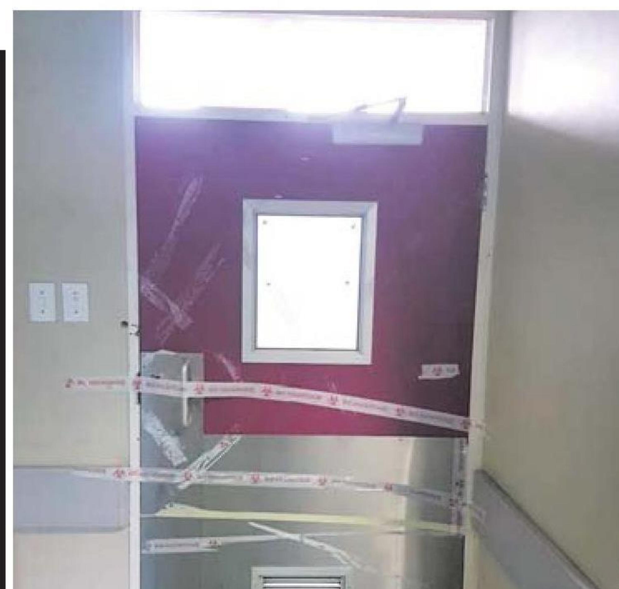
This staff bathroom is sealed-off with bio-hazard tape at Ermelo Provincial Hospital. (Photo: Supplied)
