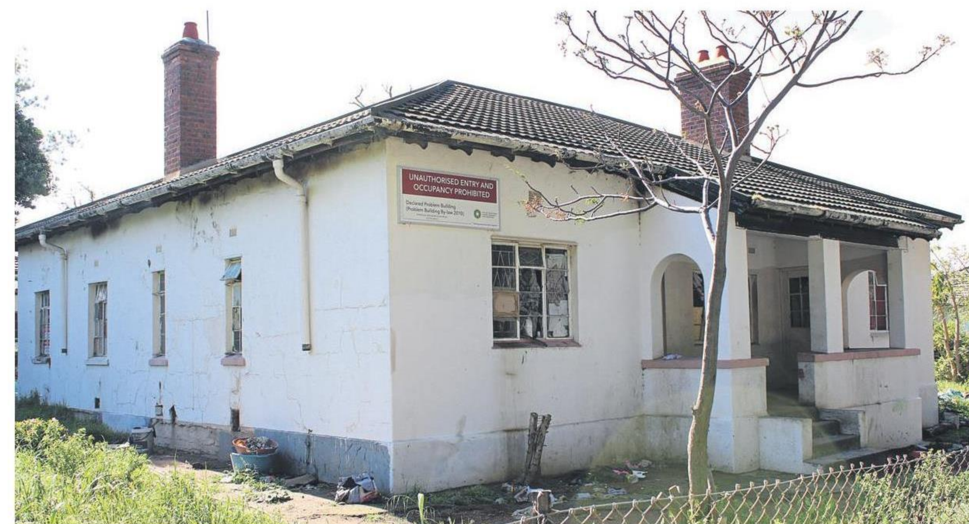
This problem building in Andries Pretorius Street, which belongs to the national Department of Public Works, has been occupied unlawfully for three years and continues to be a risk factor to the community. Photo: Yaseen Gaffar
