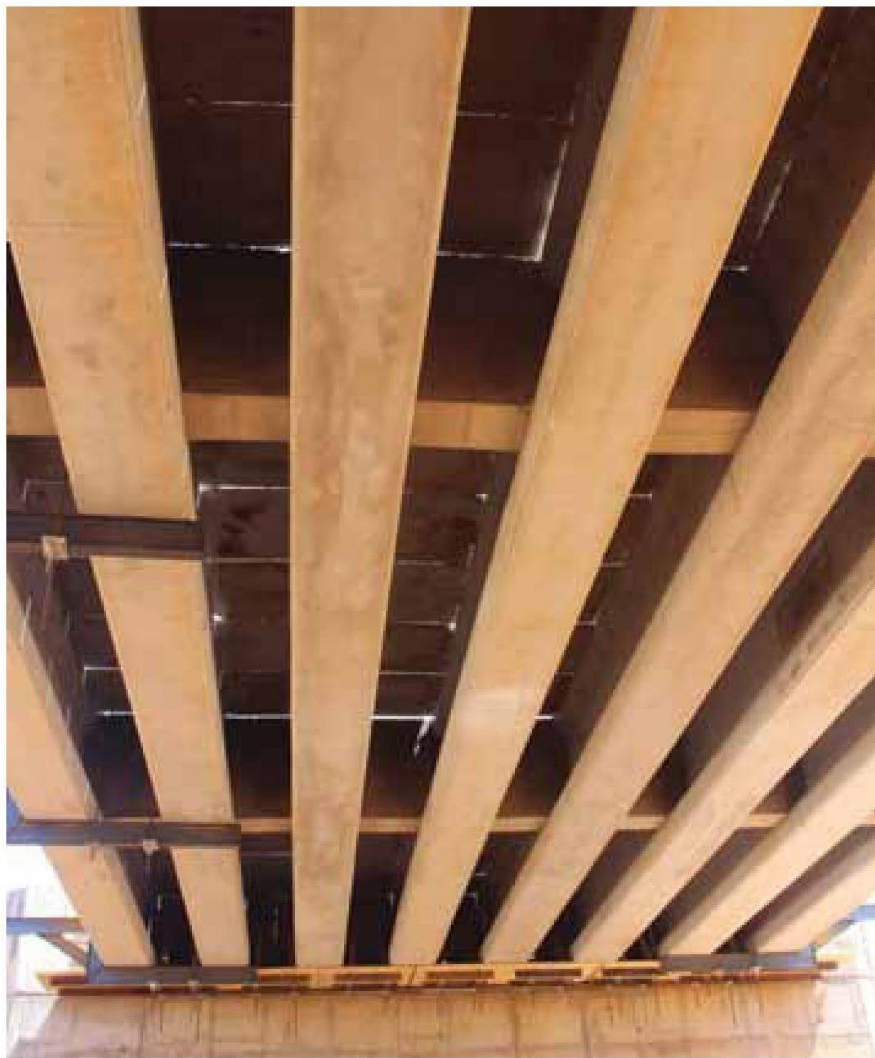
The eight 18 precast-concrete beams and 126 precast concrete deck planks were manufactured and installed by CoreCivils, the precast-concrete bridge beam and parapet arm of CoreSlab
