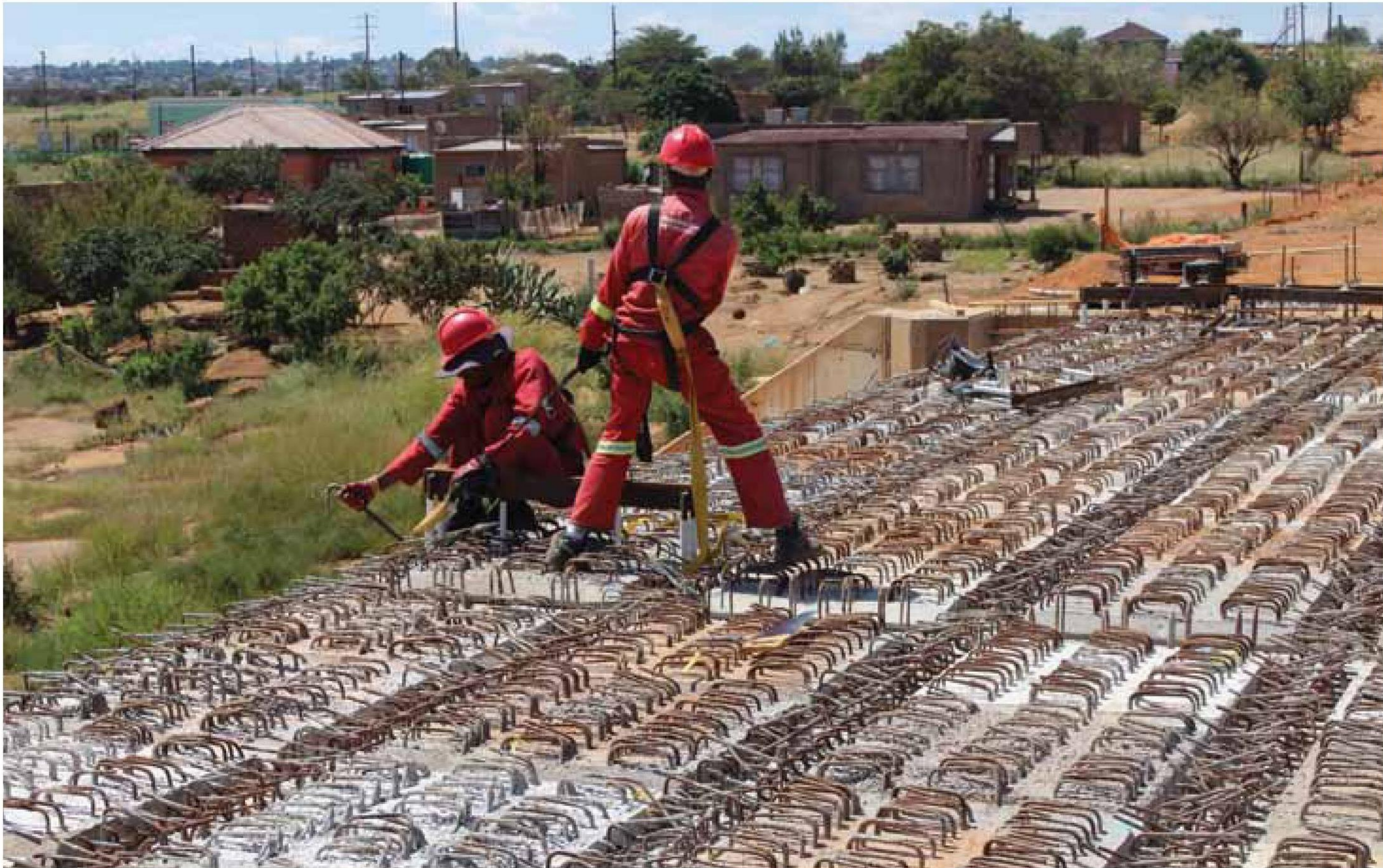
Lonerock Construction completed the bulk of the complex structural work ahead of the roadworks.
